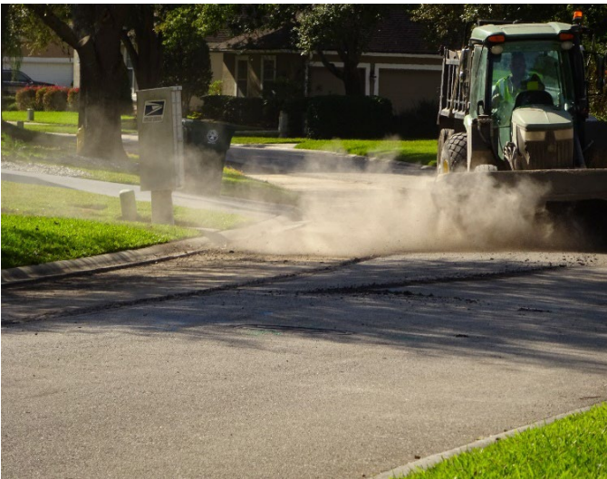
Figure A12. Dry sweeping road with rotary broom after asphalt milling prior to re-paving. Photo by NIOSH.
