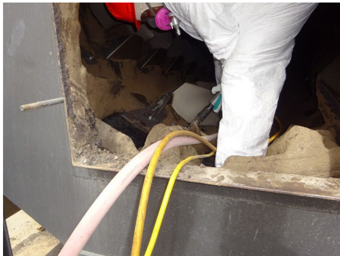
Figure A6. Worker using a pneumatic chipping hammer to remove buildup off vanes inside mixing drum. Photo by NIOSH.
