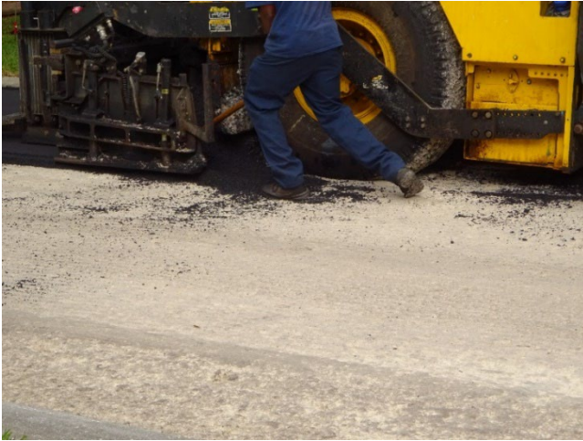
Figure A14. Paver/screeder machine laying down asphalt over freshly-milled road surface. No observable dust generated during this task. Photo by NIOSH.
