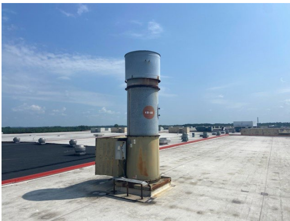
Figure B1. Exhaust stack for the 4-roll local exhaust ventilation system. Photo by NIOSH.
