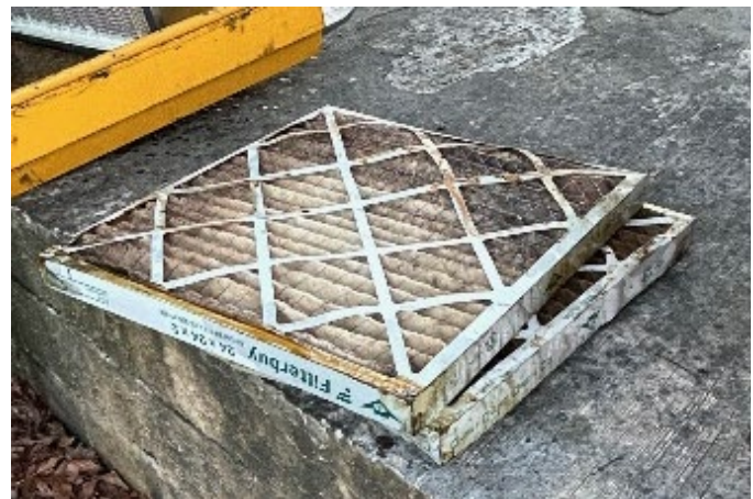
Figure B9. Dirty pre-filter. Photo by NIOSH.
