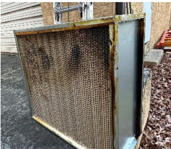
Figure B8. Dirty HEPA Filter. Photo by NIOSH.
