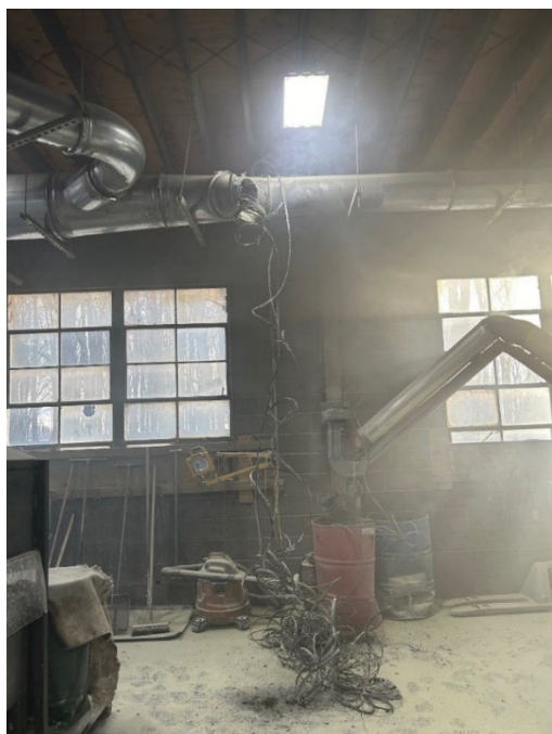
Figure B10. Ventilation ductwork after catching fire. Photo by NIOSH.
