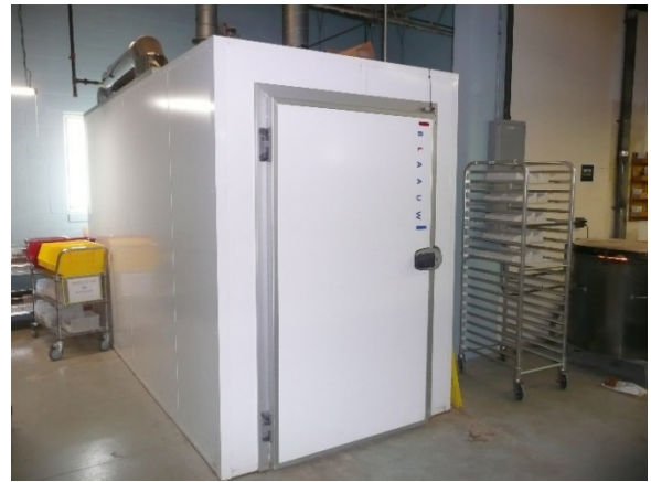
Figure 7. Enclosed gas-fired dryer.
