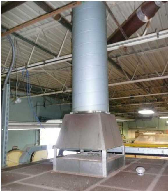
Figure 10. Rigid metal exhaust duct on top of the gas-fired kiln that extends through the roof.
