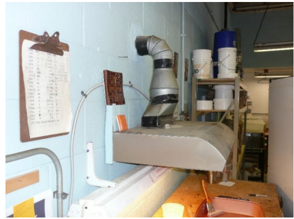
Figure 4. The hood over the paraffin wax dipping station with a 90° bend in the metal exhaust duct.
