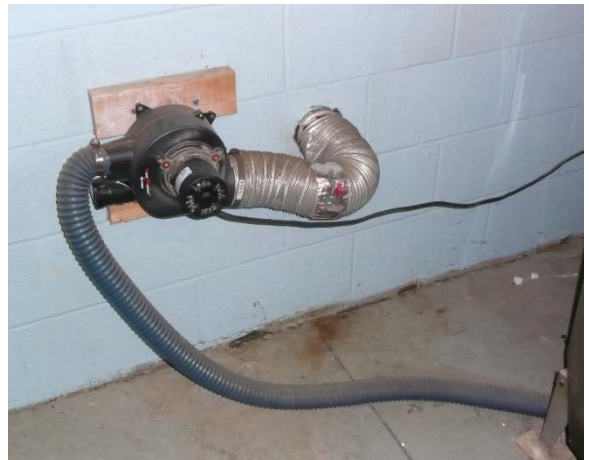
Figure 11. Flexible metal exhaust duct on an electric kiln. The duct has a sharp 90° bend and is patched with duct tape.
