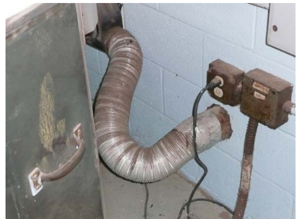
Figure 2. Excess flexible metal exhaust duct.
