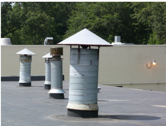
Figure 1. Rooftop capped metal exhaust stack for gas-fired kiln.
