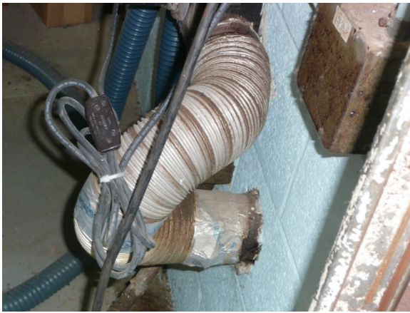
Figure 3. Flexible metal exhaust duct with a sharp bend and patched with duct tape.
