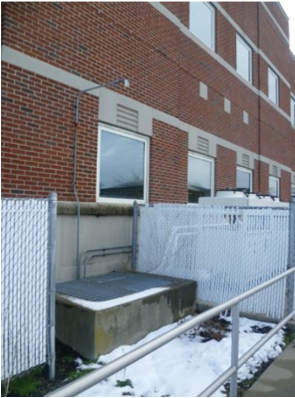
Figure A7. Outdoor air intake for MRI Suites ventilation unit, which was at grade. Photo by NIOSH.
