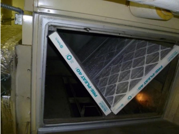
Figure A8. The filters for the MRI Suites ventilation system were tight-fitting and in a V-pattern. Photo by NIOSH.
