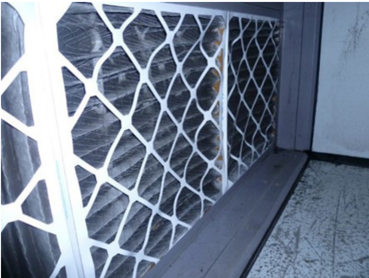
Figure A4. First bank of filters showing that the filters were bent, poorly fitting, and had damaged filter frames due to moisture. Photo by NIOSH.
