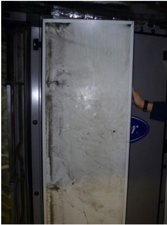
Figure A5. Door for second filter bank showing particles that had by-passed the filters. Photo by NIOSH.
