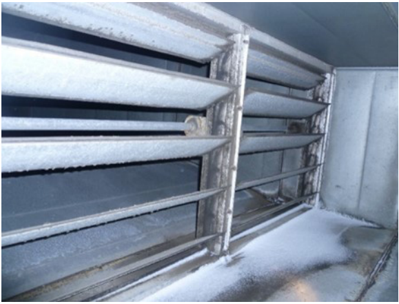
Figure A3. Snow on the downstream side of the outdoor air intake louvers of the Radiology Department HVAC unit. Photo by NIOSH.
