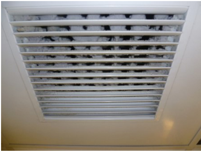
Figure A9. The supply vent shows a gray fibrous material inside the louvers. Photo by NIOSH.
