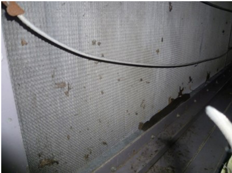
Figure A6. Debris including pieces of plant material on the cooling coils after the two banks of filters. Photo by NIOSH.
