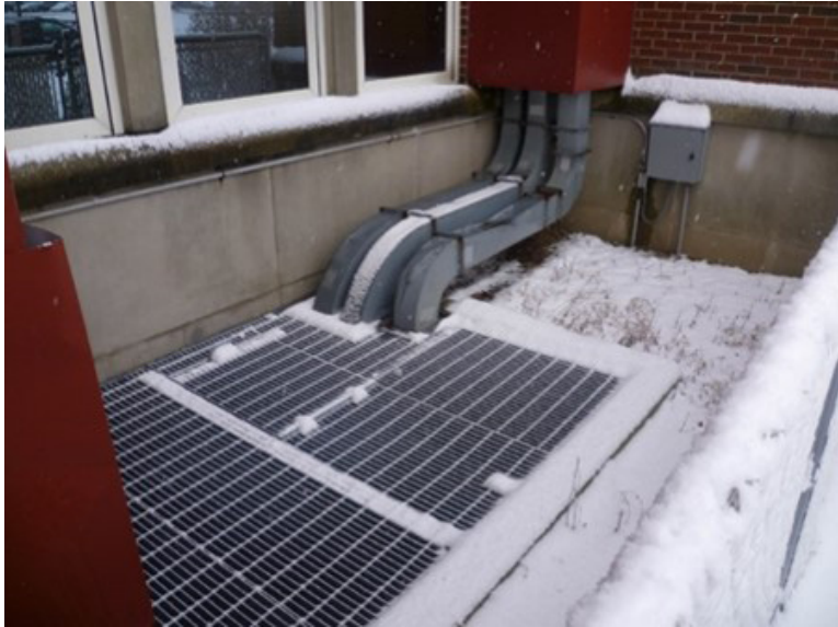
Figure A1. Outdoor air intake for Radiology Department ventilation unit, which was below grade. Photo by NIOSH.
