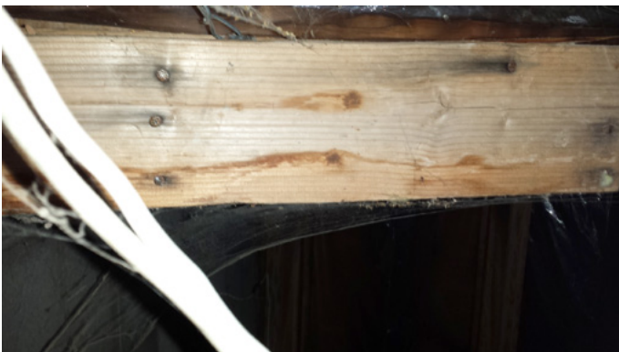
Figure 9. Water staining on a wooden beam above the ceiling tile in the owner's office, NIOSH survey, February 2016.
