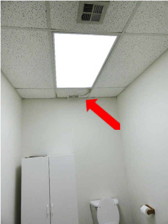
Figure 8. Water stain on the ceiling tiles around the exhaust fan above the toilet in the restroom, NIOSH survey, February 2016.
