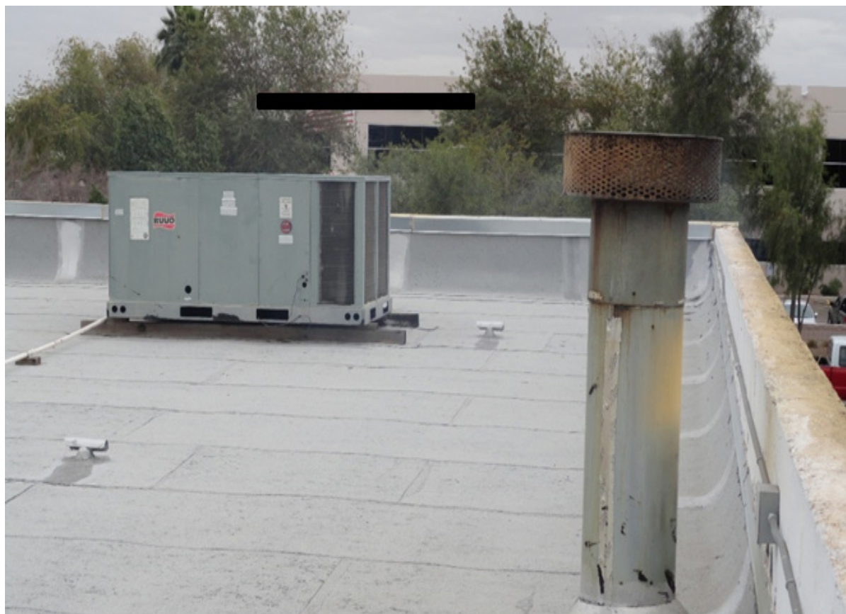
Figure 1. Roaster exhaust stack partially obstructed by chaff and debris, NIOSH survey, February 2016.
