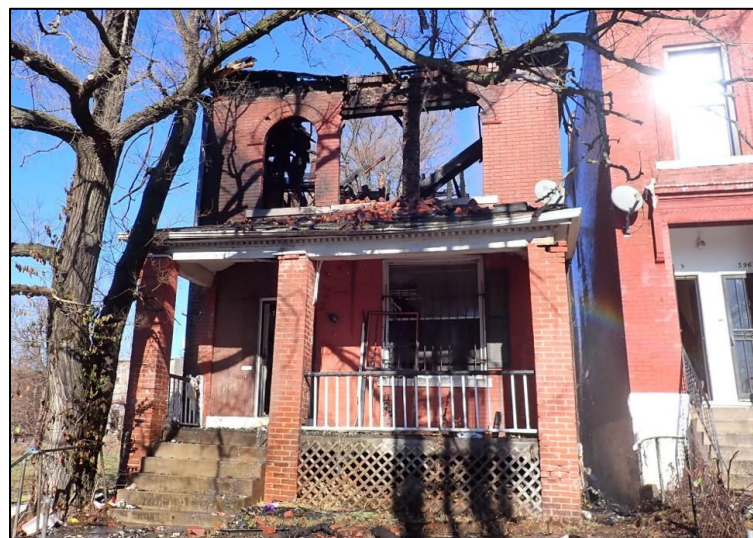
Side Alpha post fire conditions. Photo courtesy of FD.
