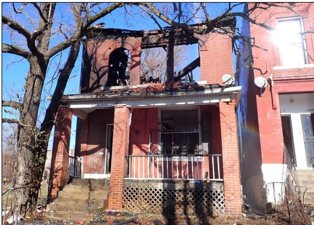
Photo 3. Side Alpha post fire conditions. (Courtesy of FD)
