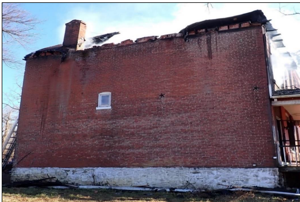
Photo 4. Side Bravo post fire conditions. (Courtesy of FD)
