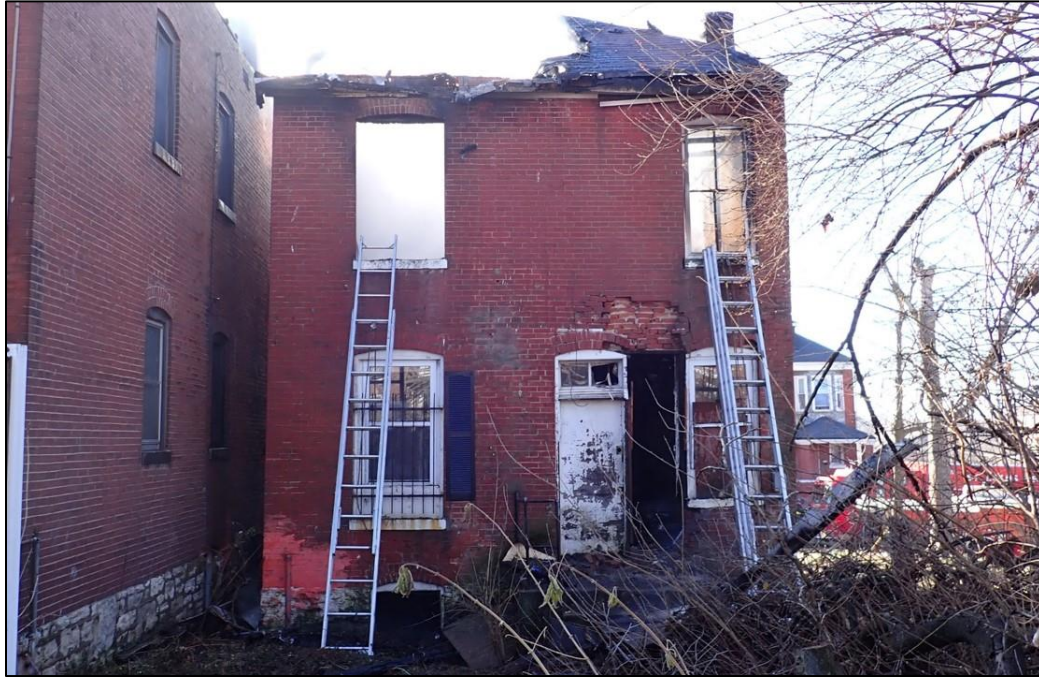
Photo 5. Side Charlie post fire conditions showing the missing wall section on the 1 st floor and the basement window used to access the basement by a member of RS-2. (Courtesy of FD)
