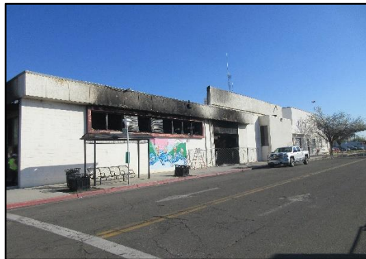
Photo 2: Fire structure Side Alpha (Photo by NIOSH)
