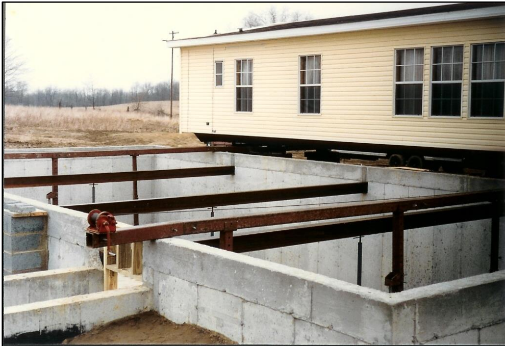
Photo 1. An example of a modular home being placed on the foundation with a basement.
