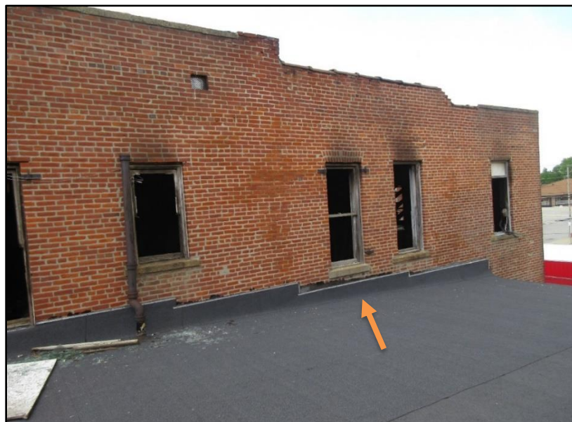
Photo 8. The Delta Exposure 1 first floor roof. The third window from left was used by RIT to recover firefighter.
