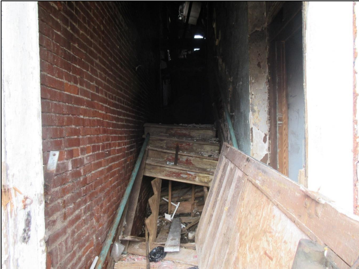
Photo 6. The stairwell against Side Charlie where the lieutenant and firefighter made entry to 2nd floor. The lieutenant was rescued by RIT underneath of the stairwell.
