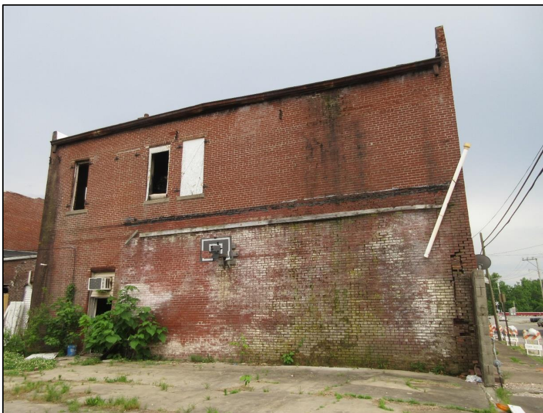
Photo 7. Side Charlie door with A/C unit over top of it. The stairwell landing to 2 nd floor that collapsed is just above door and A/C unit inside the wall.
