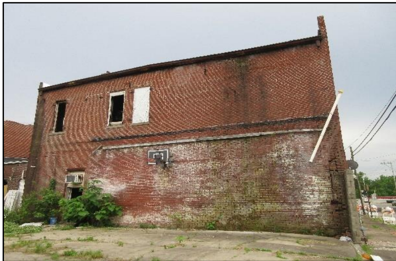
Photo 3. Side Charlie of the fire building (NIOSH photo)
