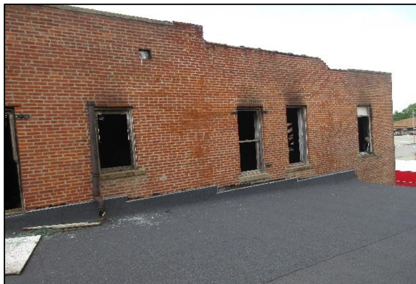
Photo 4. Side Delta, 2 nd story of the fire building. (NIOSH photo)
