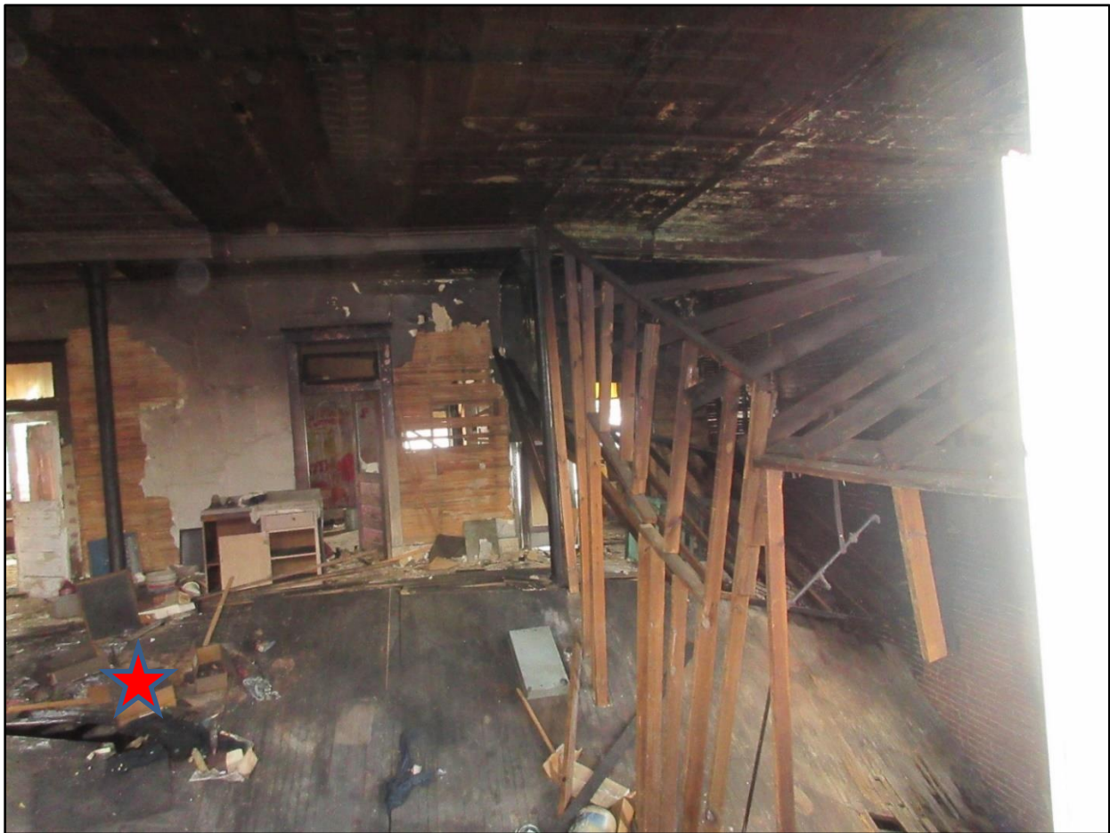
Photo 9. A view of the 2 nd floor from Delta 1 Exposure roof. Note the hole in the Side Charlie/Side Delta corner. The red star indicates the approximate location of downed firefighter.
