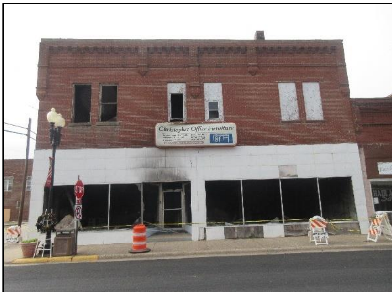
Photo 1. Side Alpha of the fire building. (NIOSH photo)
