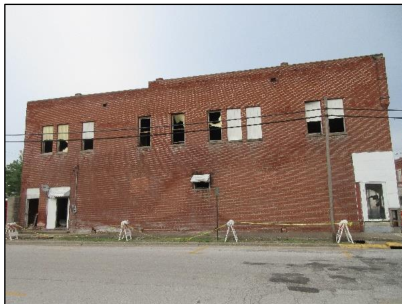
Photo 2. Side Bravo of the fire building. (NIOSH photo)
