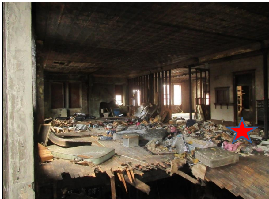
Photo 10. A view of the 2 nd floor looking from Side Charlie/Delta corner to the Side Alpha/Side Bravo corner. The hole in the floor is approximately 10 feet x 25 feet on Side Charlie/Side Delta corner where the stairwell was located. The downed firefighter (indicated by red star) was located approximately 10 feet to the right of the mattress near the right corner of the hole.
