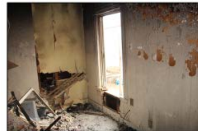
Diagram 9: Diagram and pictures of the fire room where the firefighter from Ladder 4 (L403) was removed. Also see Photo 6. (Photos courtesy of the fire department.)
