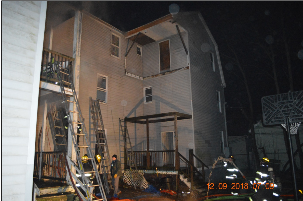
Photo 4: Decks on the 2 nd floor and 3 rd floor on the Side Bravo and Side Charlie were removed before the fire.
