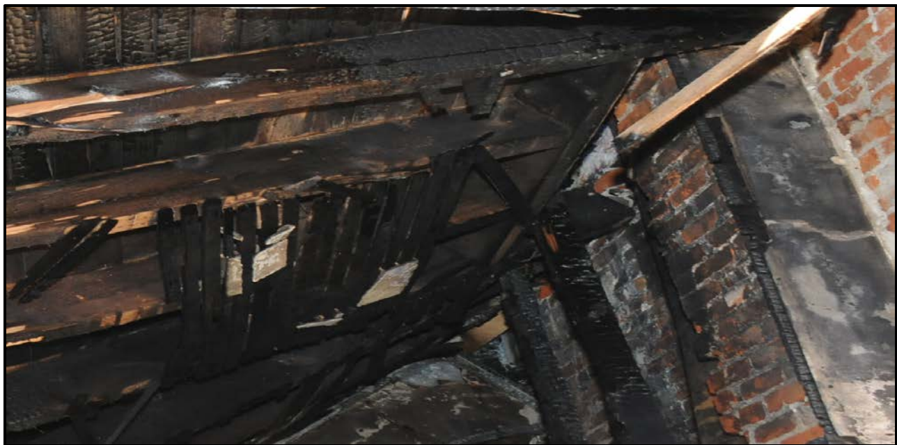
Appendix 2 Photo 10. Second Floor Collapse of Floor Joists at Fireplace. Photo Courtesy of Fire Department.
