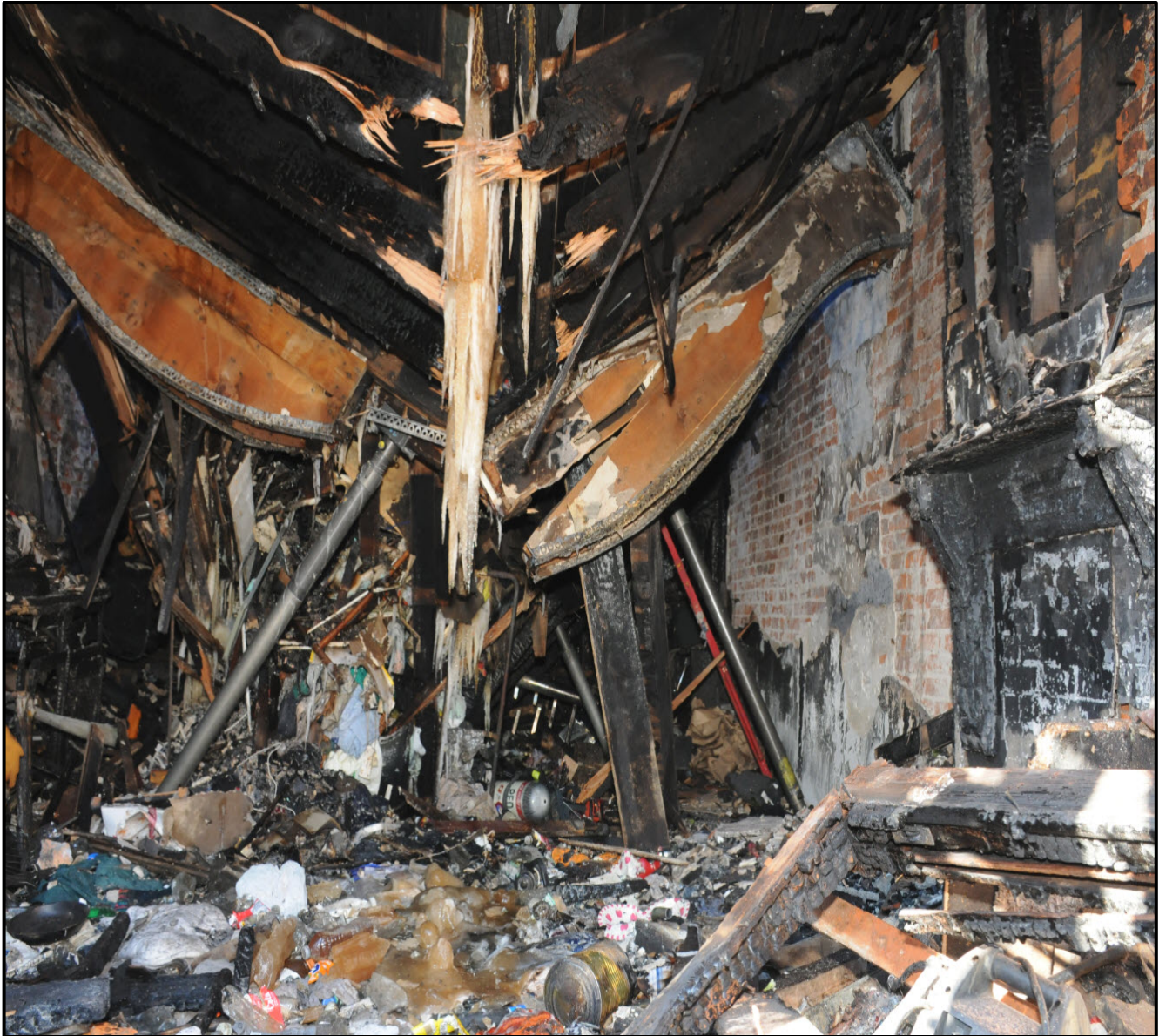
Appendix 2 Photo 6. Front First Floor Looking inward to Collapse Zone and Second Floor Debris Heavy Content. Photo Courtesy of Fire Department. Foreground: Compromised front 2 nd Floor Bedroom joists V-pattern. Background: Beyond the decorative wood “beam” is the catastrophic full V-pattern collapse of the Center 2 nd Floor Bedroom
