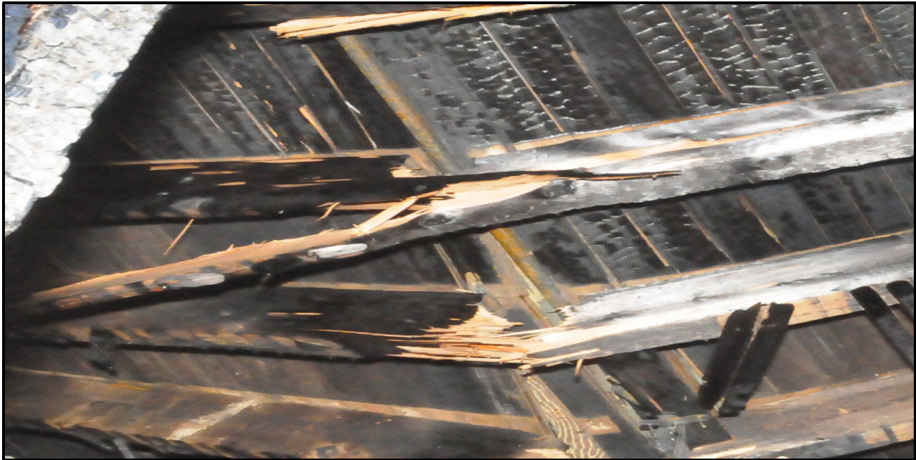
Appendix 2 Photo 9. Second Floor Collapse of Floor Joists. Photo Courtesy of Fire Department .
