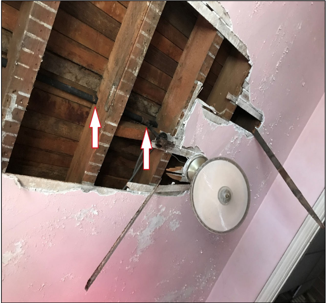
Photo 2. Exposure row house exemplar photo showing the floor joists cut to allow for gas pipe and the gas pipe drop for the light fixture. Electric light fixtures were attached to these pipes in later years.
