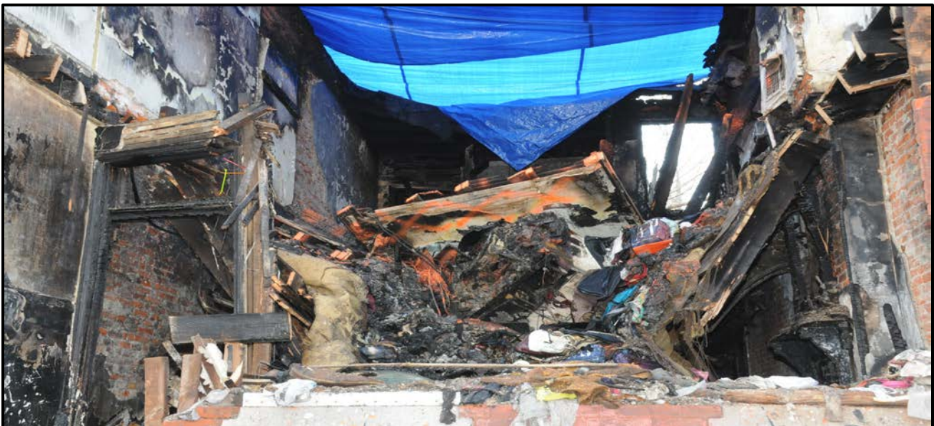
Appendix 2 Photo 8. Second Floor Collapse of Floor Joists. Photo Courtesy of Fire Department.
