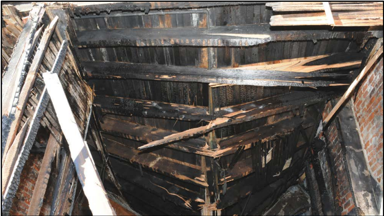
Appendix 2 Photo 7. Front First Floor Looking inward to Collapse Zone and Second Floor Debris Heavy Content. Photo Courtesy of Fire Department.
