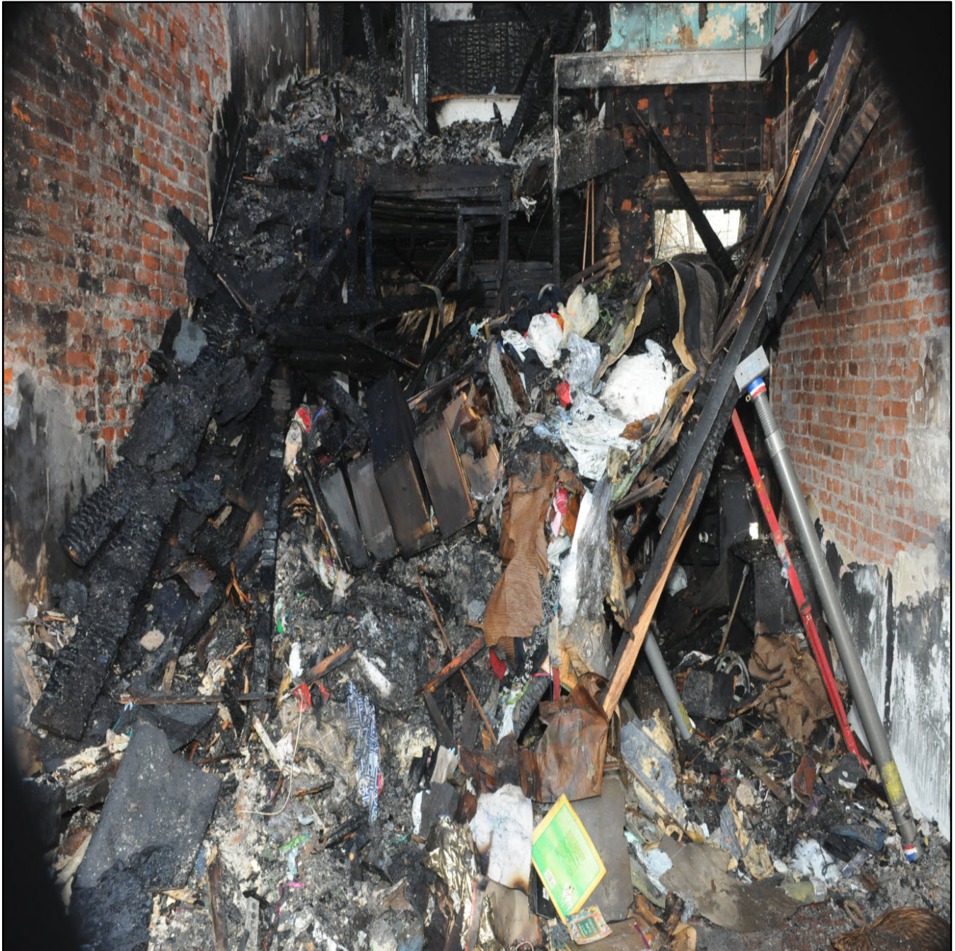
Appendix 2 Photo 5. Front First Floor Looking inward to Collapse Zone 1 st Floor. Photo Courtesy of Fire Department. Hoarding, Heavy Content and Clutter from Second Floor Rooms into the V-Shaped Floor Collapse. Photo Courtesy of Fire Department.
