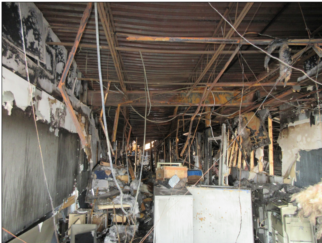
Photo 2. Interior of Side Delta exposure (computer business), looking from Side Alpha to Side Delta. Note roof support features including lightweight metal bar joists running from front to back supporting corrugated metal roof decking.
