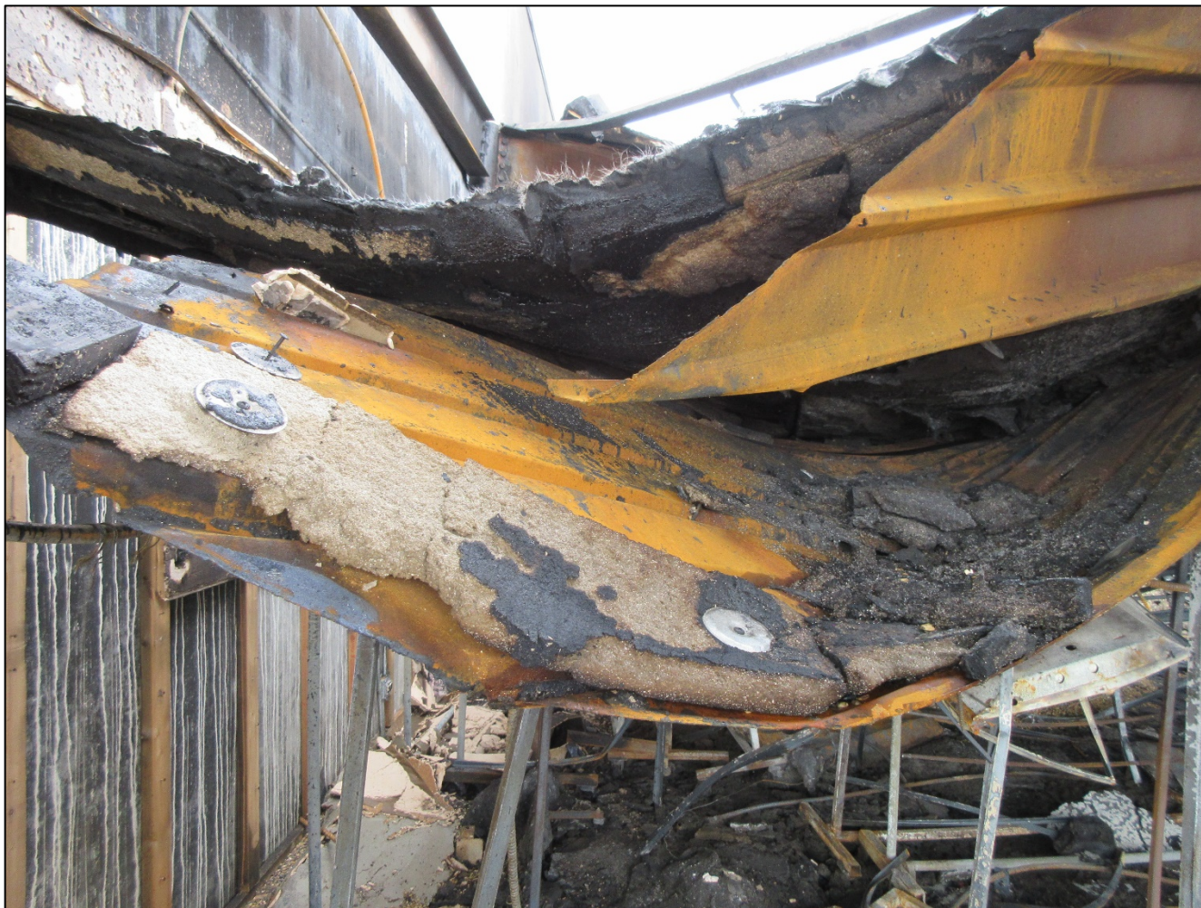
Photo 3. Close-up showing construction features of flat metal roof. Note layers of foam, waterproof membrane and asphalt. (NIOSH Photo)
