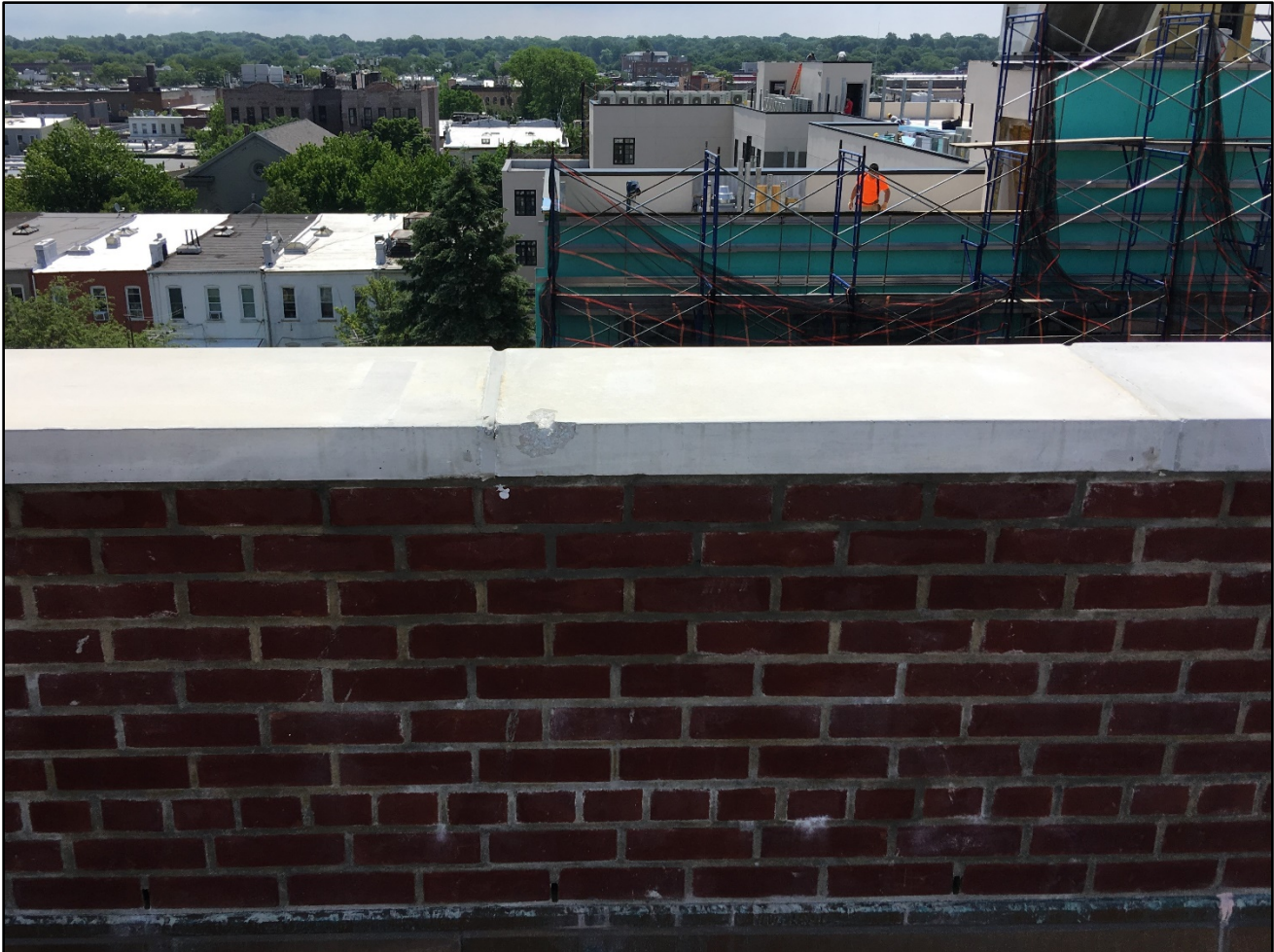
Photo 2. The parapet wall on the roof of the fire building. The height of the parapet wall is 41 inches including its concrete cap. (NIOSH Photograph.)
