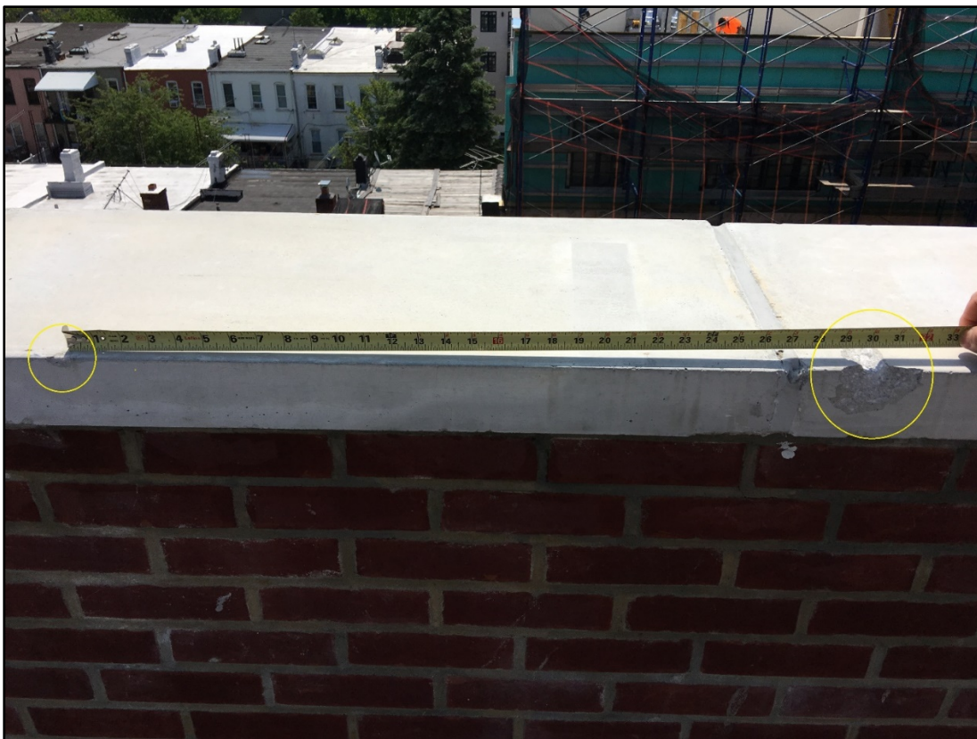
Photo 3. The yellow circles indicate the damage caused by the brackets on the bottom of TL135 when the platform came loose from the parapet wall. (NIOSH Photograph.)
