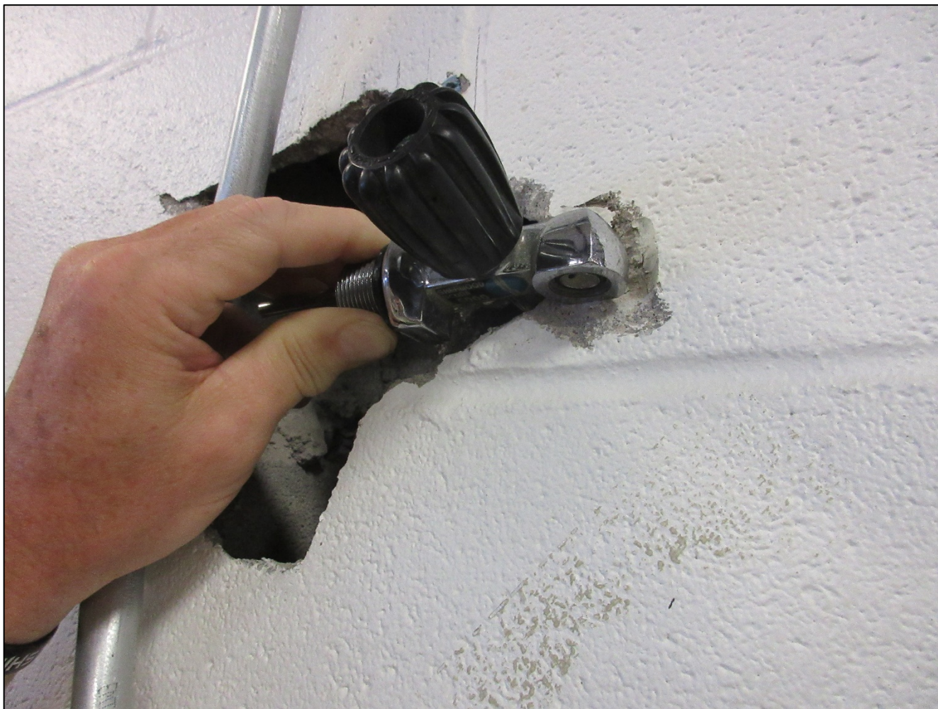
Photo 3. Exemplar SCUBA cylinder valve is held up against wall where the incident SCUBA cylinder struck the engine bay wall, creating a hole in the wall. Note how the shape of the cylinder valve matches the damaged area on the wall
