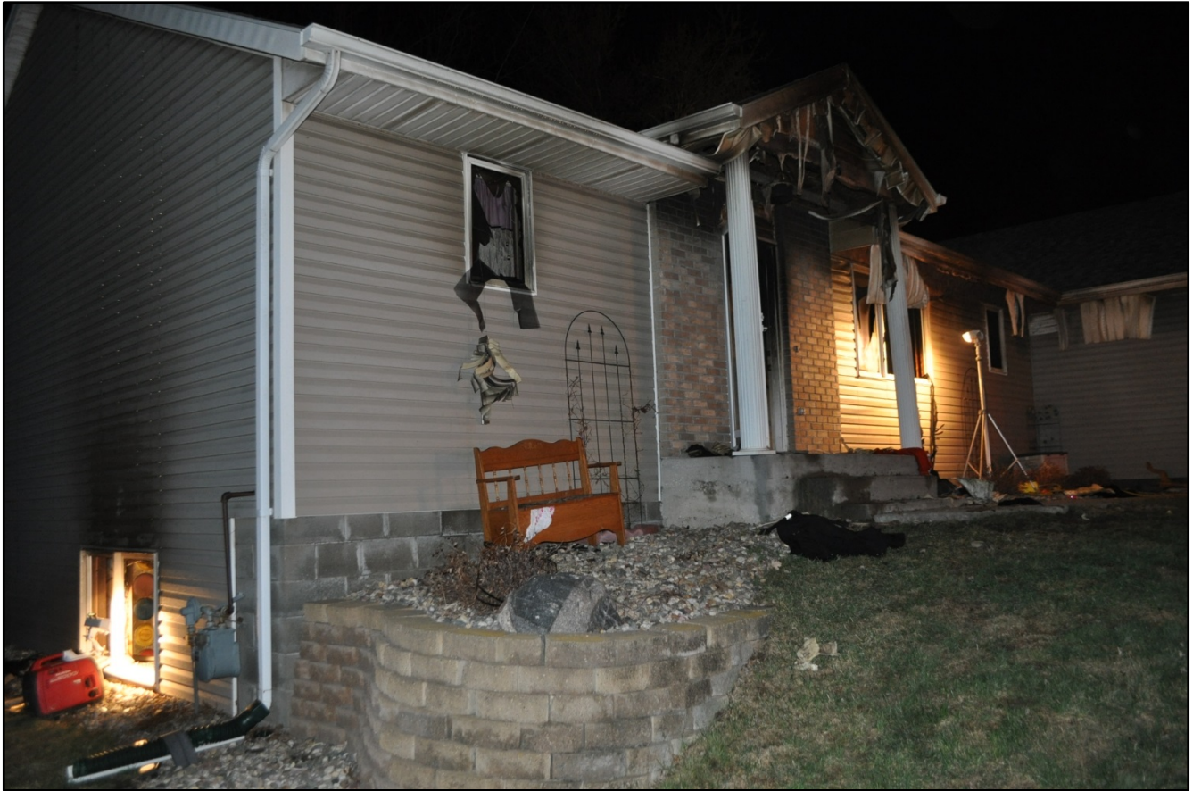
Photo 1. Front, side A, view of fire structure. (Courtesy of the Fire Marshall's Office.)
