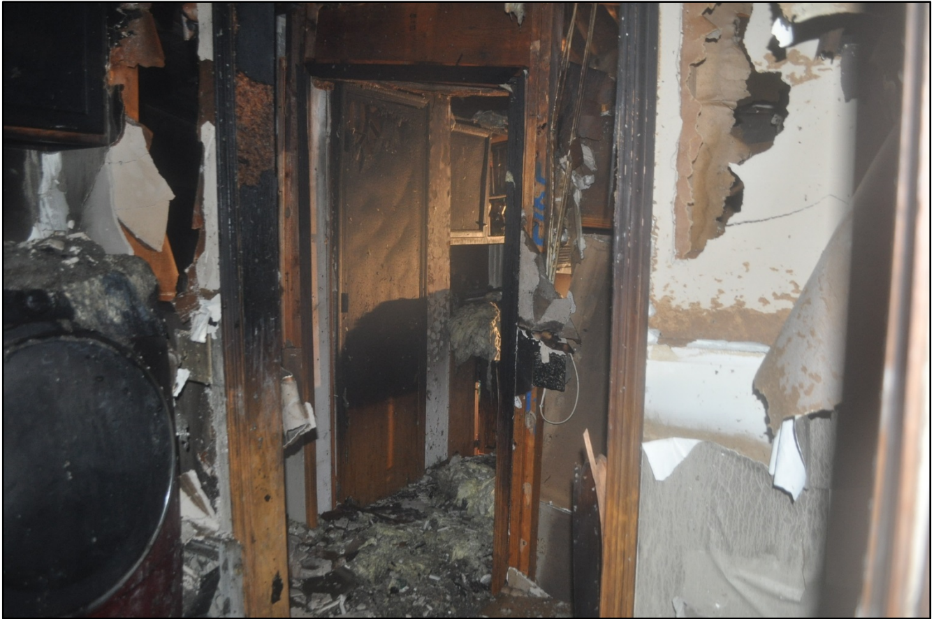
Photo 3: View from laundry room across hallway into the kitchen. (Courtesy of the Fire Marshall's Office.)
