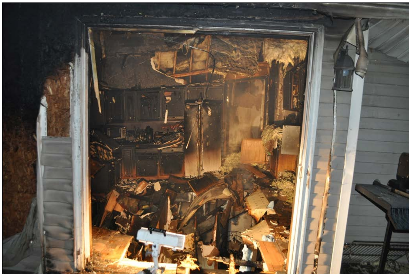
Photo 4. View from rear sliding doors looking into the kitchen and the floor collapse in the kitchen area. The entry into the kitchen is just to the right of the refrigerator. (Courtesy of the Fire Marshall's Office.)
