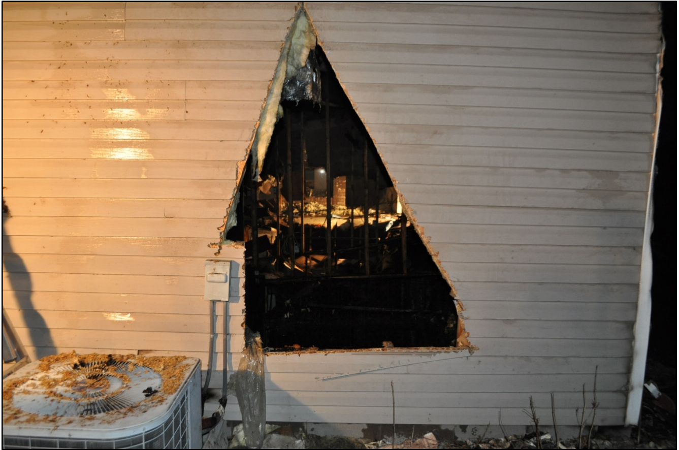
Photo 5. Initial hole cut on Side D to look for the missing fire fighter. (Courtesy of the Fire Marshall's Office.)
