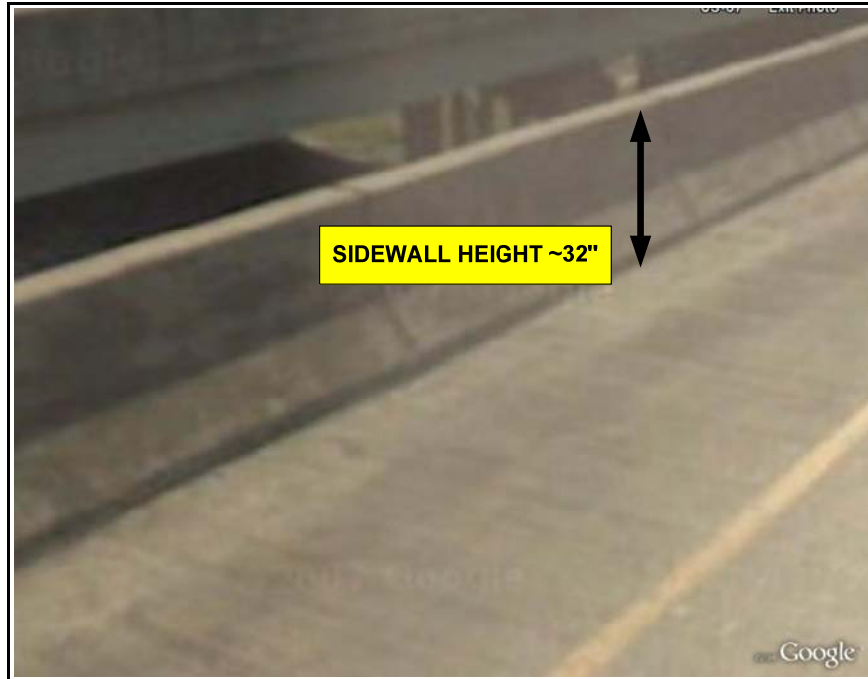
Photo 2. View of bridge sidewall at the location where the victim fell. Depiction from Google Earth
