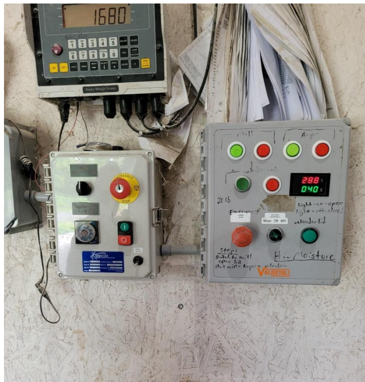
Photo 4. Unloader controls and emergency shutoff devices.
