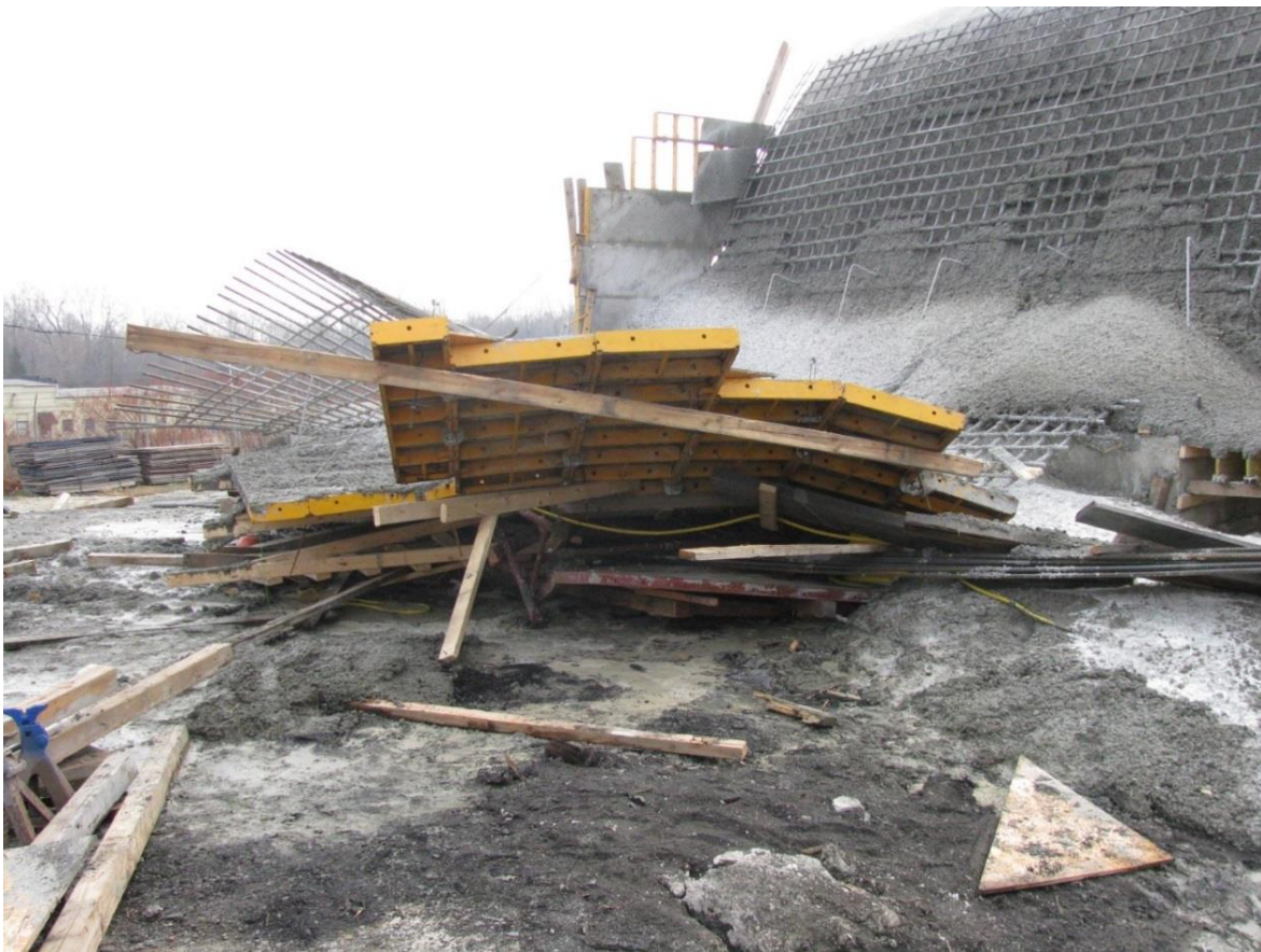
Photo 1. The site of collapsed form support of buttress section of aqueduct mockup (photo courtesy of OSHA)
