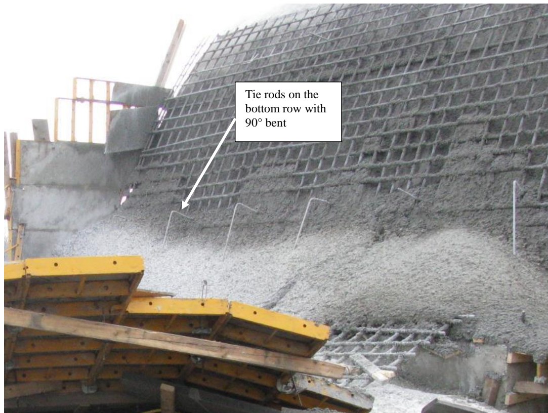
Photo 4. Tie rods that remained on the concrete bent at a nearly 90° angle suggesting a vertical drop in the retaining wall during collapse (photo courtesy of OSHA).
