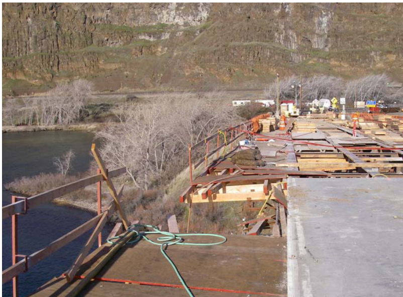
Photo 10: Site where excavator tipped over showing damage to guardrail, temporary walkway, and marks caused by excavator sliding
