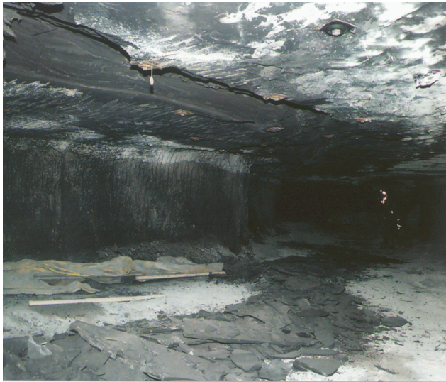
Figure 4. Stress induced cutter roof failure
