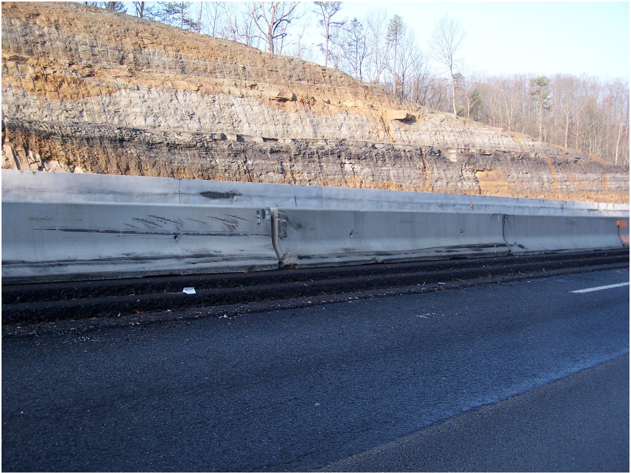
Photograph of the three temporary barrier sections semi driver struck. Marks are from the semi. Photograph courtesy of Kentucky Vehicle Enforcement.
