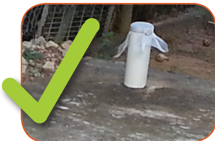
Septic tank ventilation pipe with screen mesh
