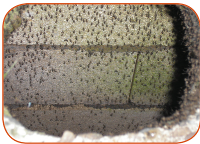
Mosquitoes in a septic tank
