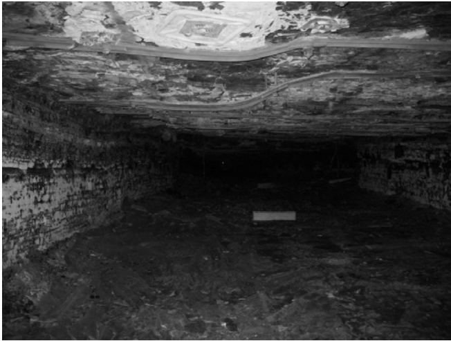
Figure 8. Photo of the rock collection area, looking inby from the intersection, taken on March 3, 2008.
