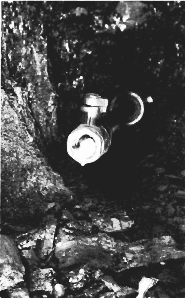
FIGURE 13. - Hole 2 five days after being grouted, location A (fig. 8). Note wet grout in the valve.
