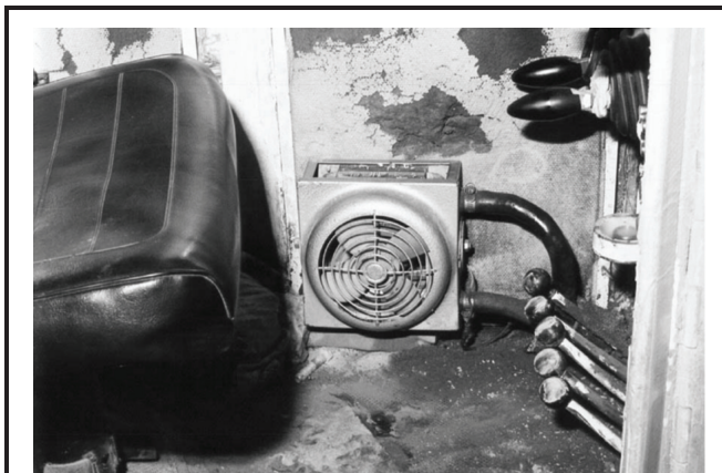
FIGURE 2. Floor heater inside enclosed cab
