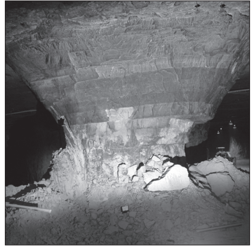
Figure 2. Pillar that had an original width to height ratio of 1.7 failed by progressive spalling. Thin weak beds are thought to have contributed to the failure. Average pillar stress is about 11% of the UCS.
