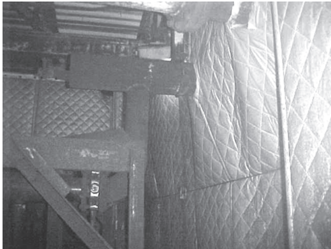
Figure 3 — Barrier-absorber curtain between Screens 169 and 167 showing tight seal around piping.
