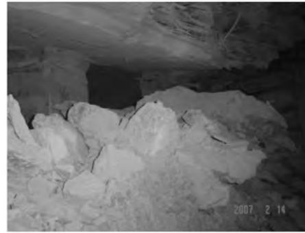
Figure 4 — Case study: poor ground conditions at a trona mine.
