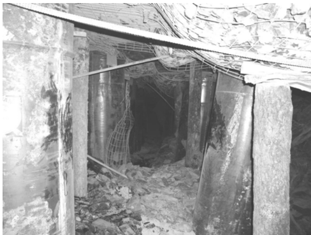
Figure 14. Response of can-supported gateroad entry to floor heave, and pillar and roof damage produced by M 1.9 coal bump.
