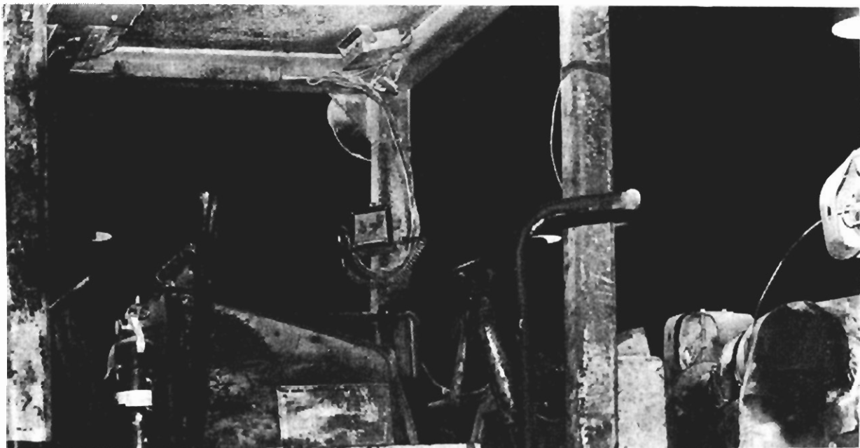
FIGURE 3.18. TYPICAL RADIO INSTALLATION IN A MINE VEHICLE SHOWING THE MODAT EMERGENCY ALARM, IDENTIFICATION AND STATUS ENCODER UNDER THE ROOF AND THE RADIO CONTROL HEAD MOUNTED ON THE COLUMN.
