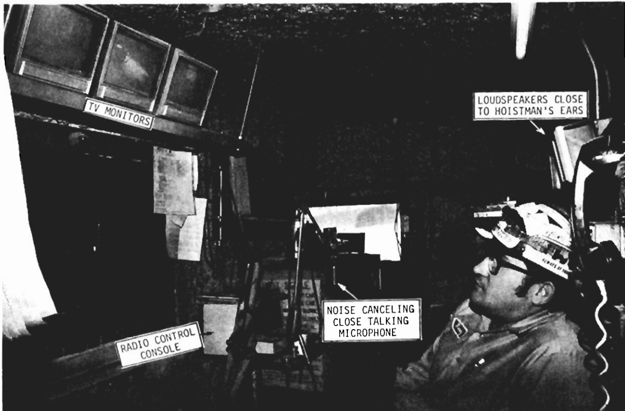
FIGURE 3.16. TV MONITORS AND RADIO CONTROL EQUIPMENT IN THE HOIST HOUSE.
