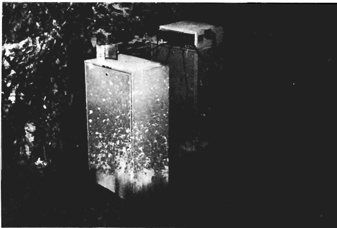
FIGURE 3.1. INITIAL INSTALLATION OF MULTIPLEXING EQUIPMENT AND BASE AND CONTROL STATIONS AT THE BASE OF THE SLOPE.
