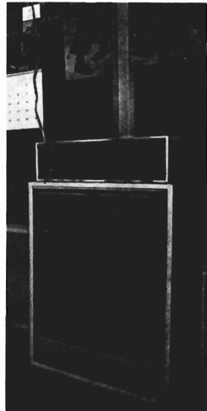
FIGURE 3.9B MODAT ALARM AND MOBILE UNIT IDENTIFICATION DECODER IN FOREMAN'S OFFICE.
