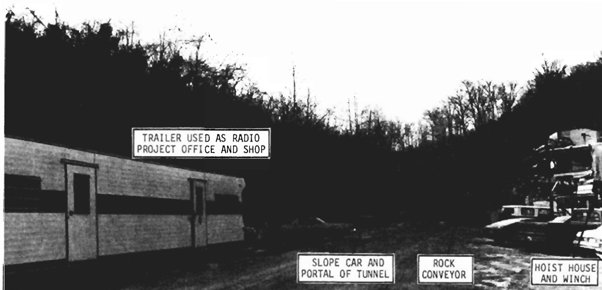
FIGURE 1.1 VIEW OF RADIO SHOP AND THE MINE PORTAL. THE MINE IS ENTERED THROUGH THE 2200 FOOT SLOPE TUNNEL WHICH HAS RAILS FOR THE SLOPE CAR AND A BELT CONVEYOR FOR CRUSHED LIMESTONE.
