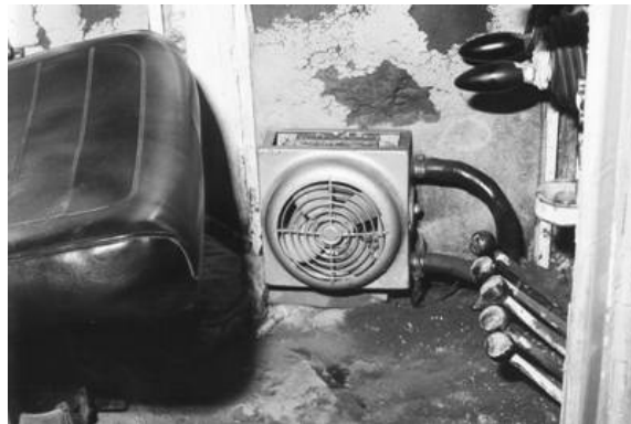
Figure 1. Floor heater in surface drill cab.
