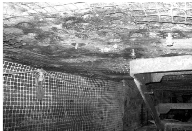
Figure 5. Bolt installation site in NIOSH Safety Research Coal Mine (SRCM), showing the 3 inch diameter holes from overcored bolts and several previously pulled bolts which were not removed from the roof
