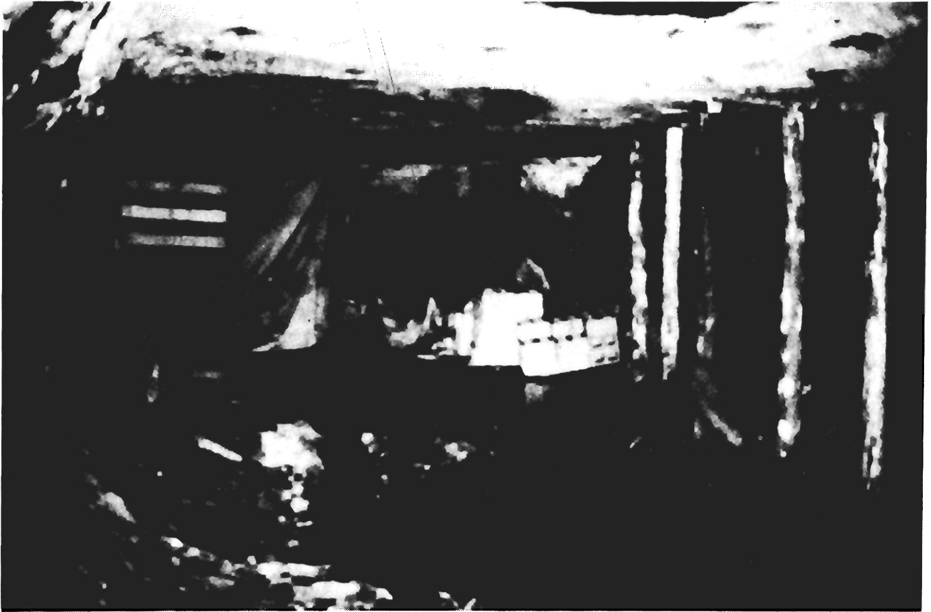
FIGURE 4.—Standing water located outby Mine B seals.
