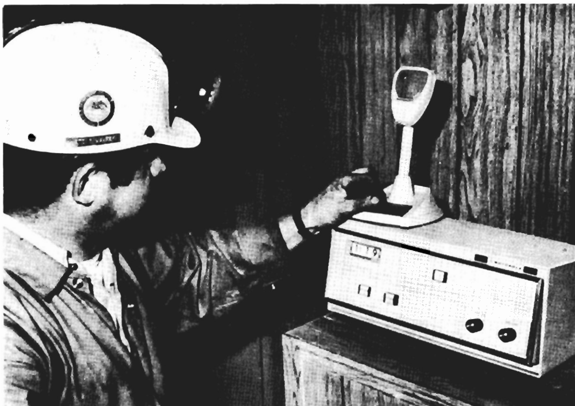
FIGURE 17. - System control console.
