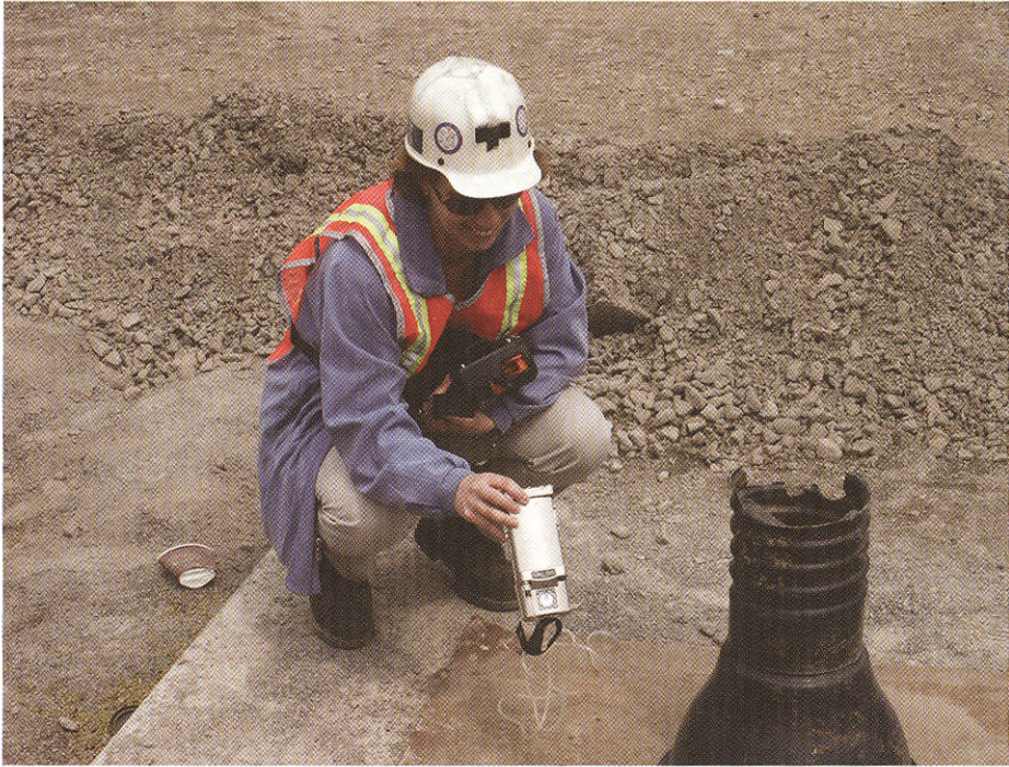
Figure 28.3 - Worker using a multi-gas monitor to measure blasting fumes in a manhole, on a trenching project. (Courtesy: R. Maimiero)
