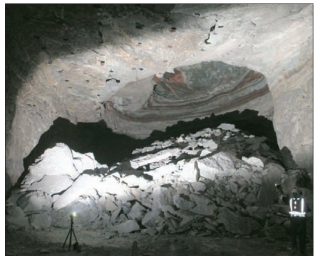
Figure 4—Large-oval shaped fall that has propagated upwards into weaker overlying strata in a limestone mine
