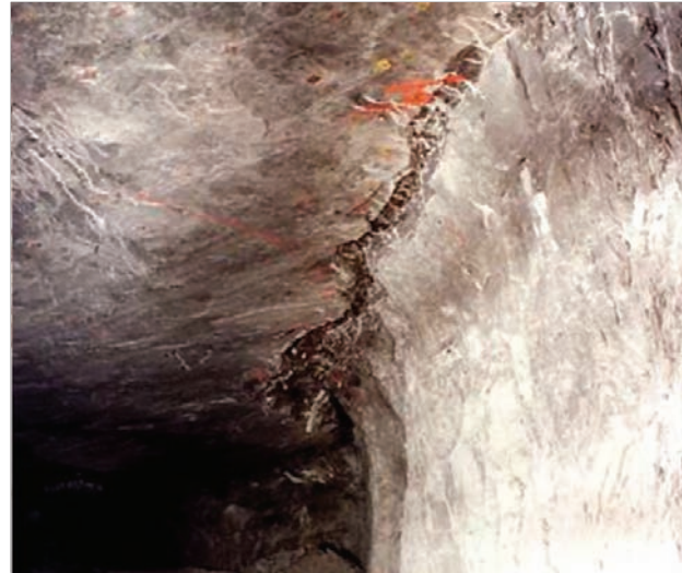
Figure 2—Roof guttering at the pillar-roof contact
