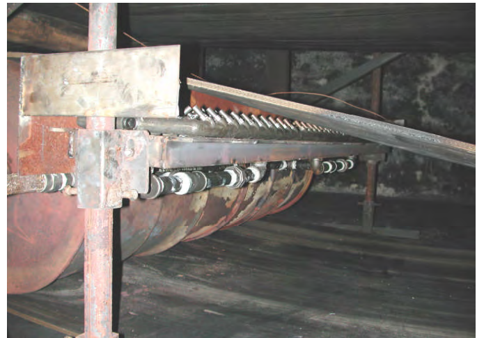
Figure 3. Natural gas burners to ignite belt.
