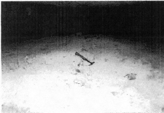
Figure 12. Floor heave experienced in E15 panel
