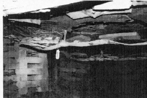
Figure 17. Rear abutment stress damage in L1 entry
