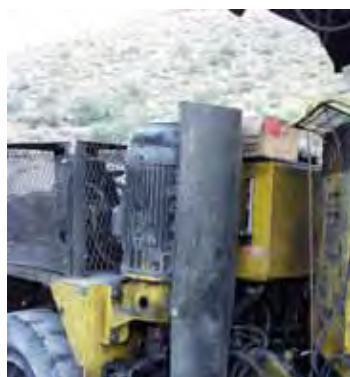
Figure 23. Heavy conveyor belt barrier.
