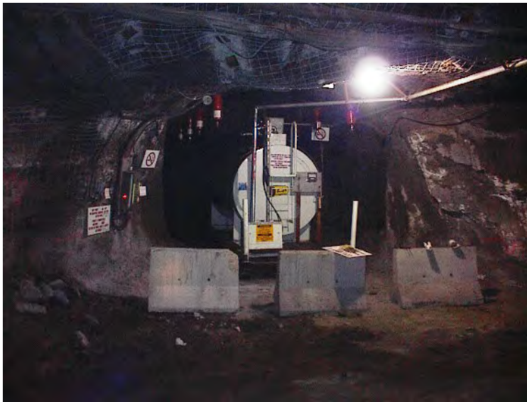
Figure 22 - Blended Fuel Storage at 1000 Level
