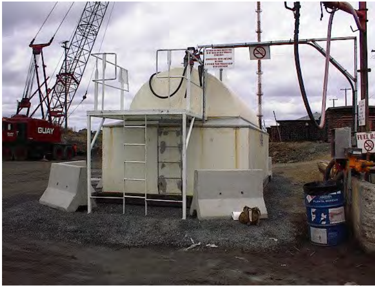
Figure 21 - Blended Fuel Storage on Surface
