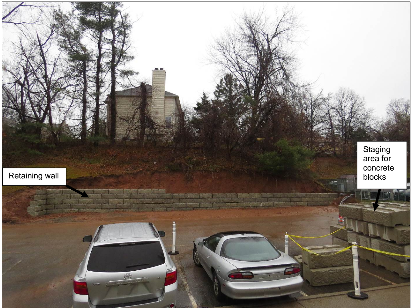
FIGURE 1. Incident site; a) parking lot of health care facility, b) closer view of retaining wall.
