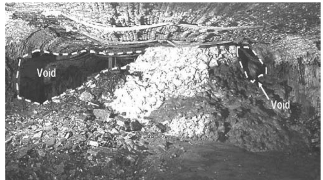
Figure 4 — Cement-based remotely installed mine seal (Urosek, 2005). Note the open void areas.
