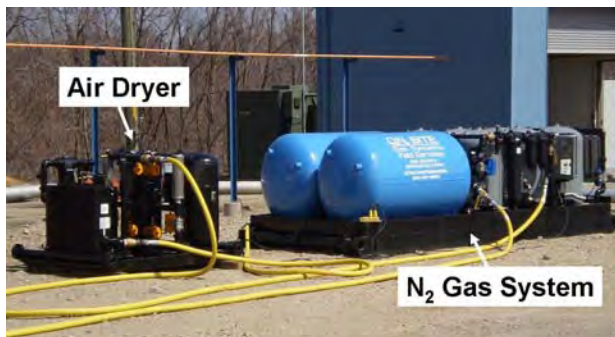
Figure 3. N 2 generating system with air dryer.
