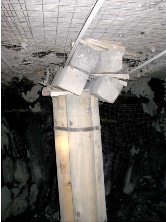
Figure 17. Adding crib timbers to the top of a Cluster Prop is not advisable. As shown in this figure, this can create a hinge point that can severely degrade the stability of the support in high deformation environments.
