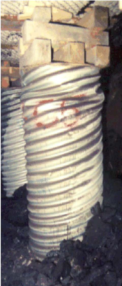
Figure 2. Confined Core Crib (3C) support was the first viable alternative to wood cribbing in western longwall tailgates.
