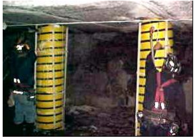
Figure 18. Pumpable roof supports offer an alternative support system whereby the support material can be pumped from the surface or a remote underground location.
