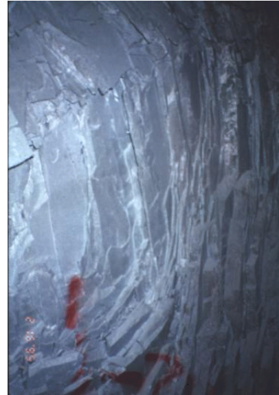
Figure 2. Edge of burst cavity shown in Figure 1. Note closely spaced fractures.
