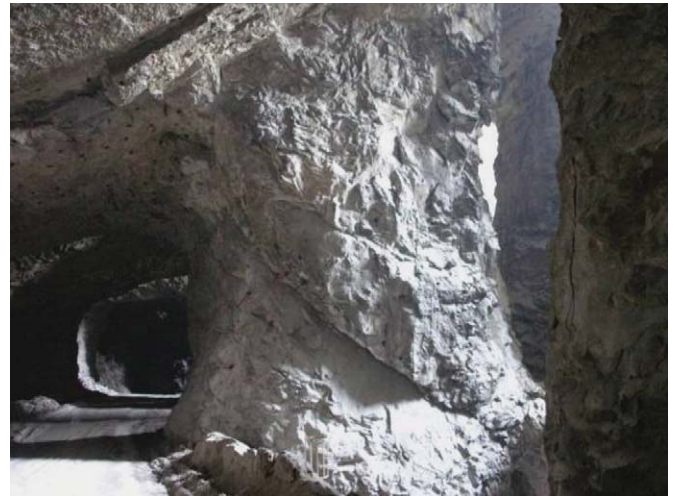
Fig. 1. Example of a pillar that is bisected by a large angular discontinuity.
