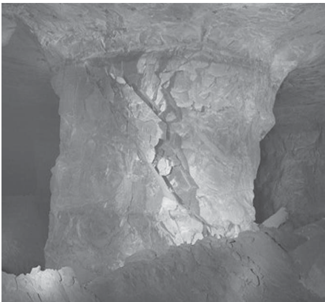
Fig. 3. Partially benched pillar that failed along two angular discontinuities. Width-to-height ratio is 0.58 based on full benching height and average pillar stress is about 4% of the UCS.
