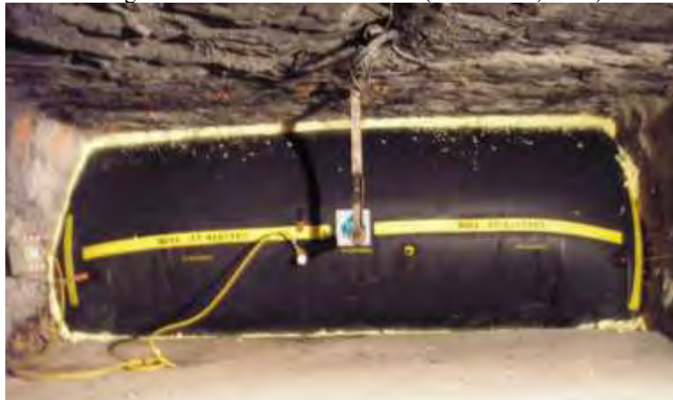
Figure 5. Underground testing of an inflatable temporary ventilation control device (Trevits et al. , 2009).
