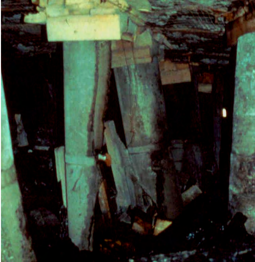
Figure 11 - Failure of concrete cribs in longwall tailgate due to convergence beyond the control of the support system.
