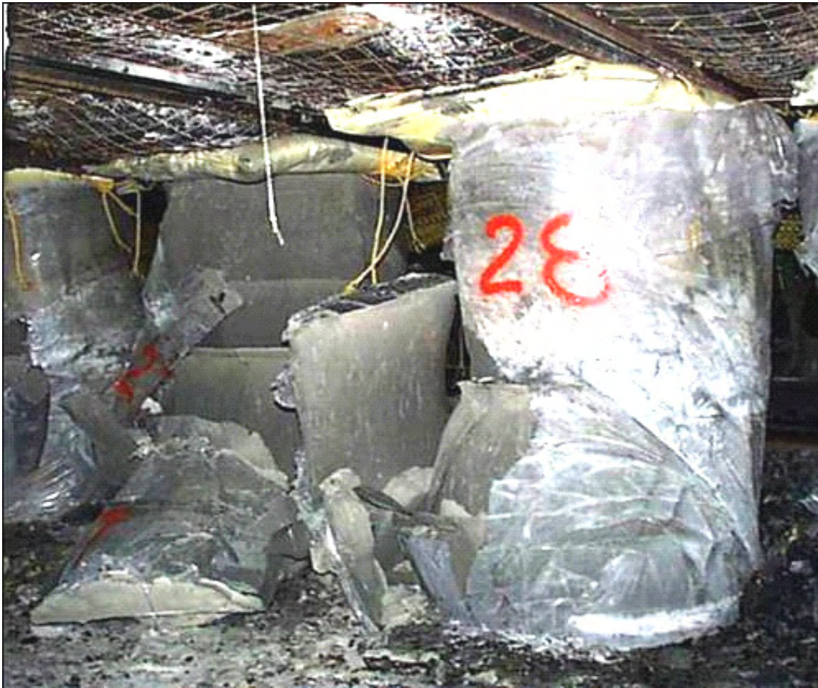
Figure 12 - Failure of pre-driven longwall recovery room support due to convergence beyond the control of the support during panel fender yielding.
